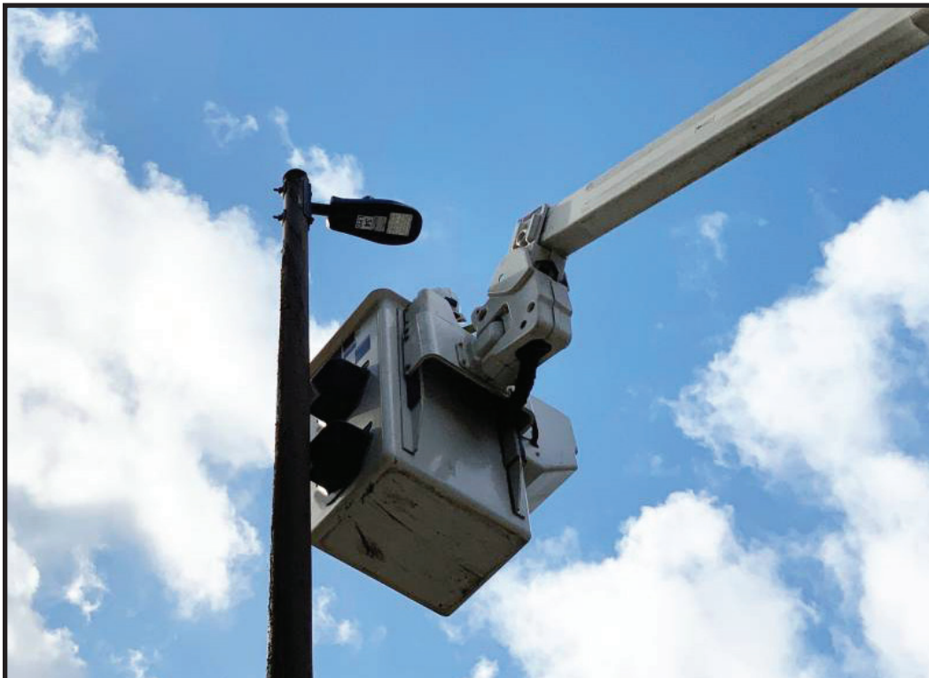
Contracted service provider PGE maintains City streetlights.
