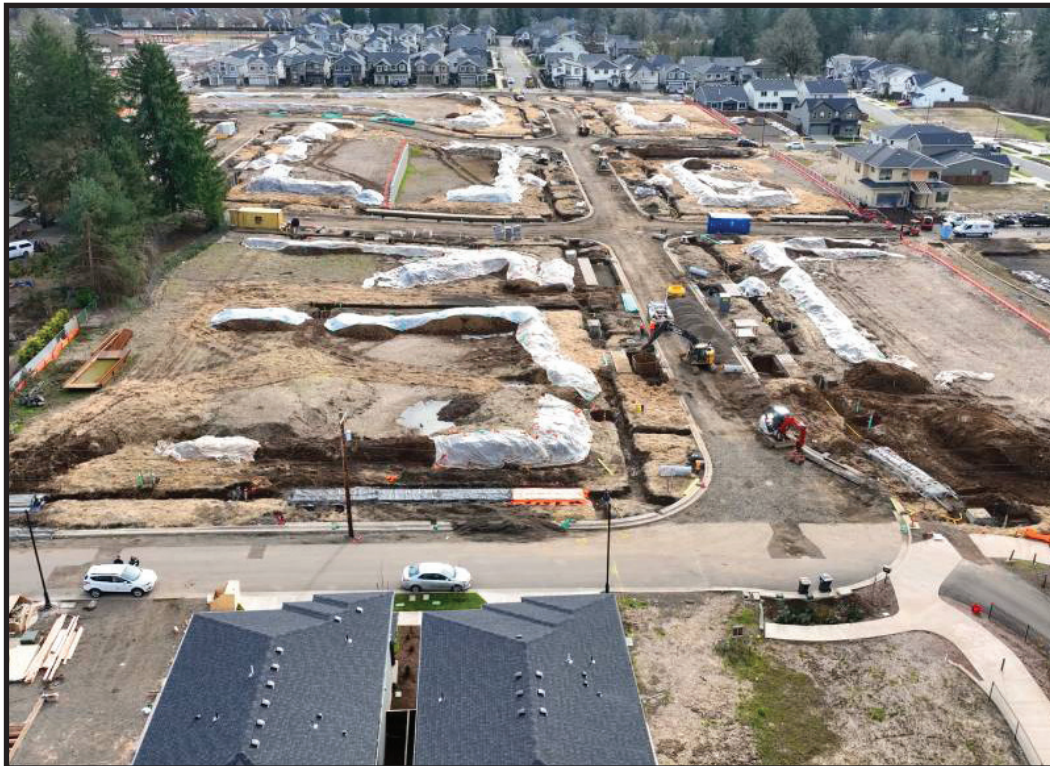
Construction of public infrastructure (streets and stormwater facilities) for the Frog Pond Ridgecrest neighborhood on January 22, 2026.
