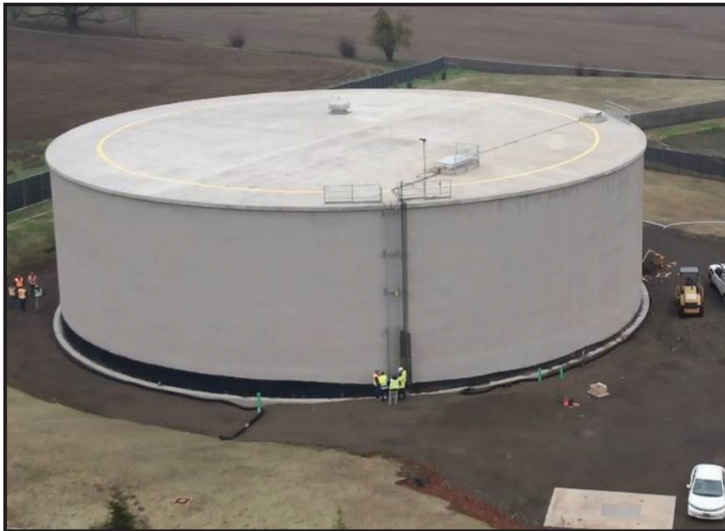
Completion of the West Side Level B Reservoir on Tooze Road (CIP #1149).
