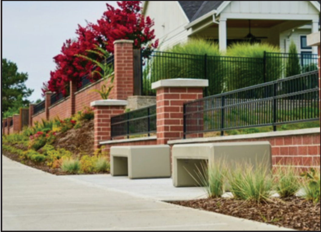
Sidewalk and Bench Installation at Meridian Creek Crossing at Boeckman Road (CIP #4205).
