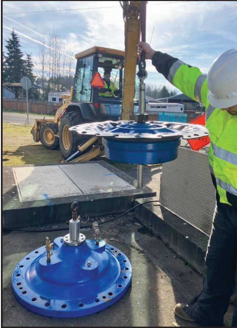
A large pressure reducing valve is serviced to prepare to bring the new Westside reservoir online.
