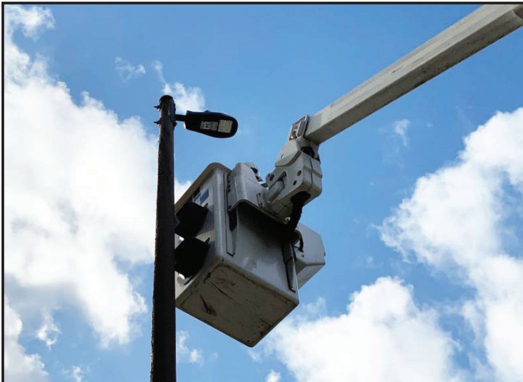
Contracted service provider PGE maintains City streetlights.
